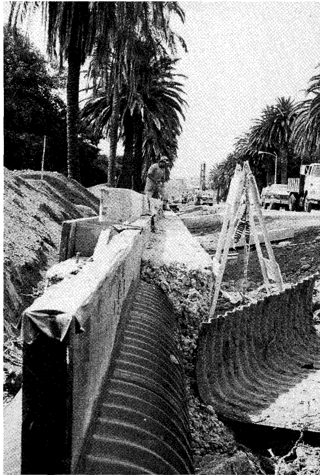
A worker lays granite curbing along Palm Drive. In left foreground is the slotted drain, covered with duct tape to keep out debris; at center, the concrete and reinforcing bar foundation for the curbing is visible.
