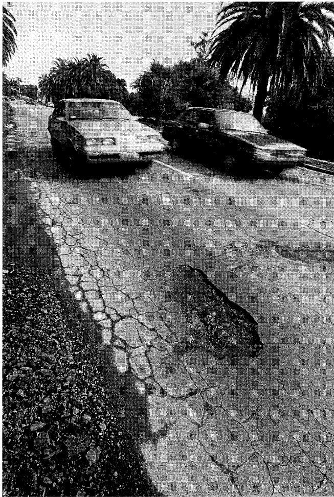
Potholes and poor drainage were among the problems corrected in the 1994 reconstruction of Palm Drive.
