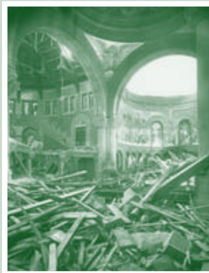
Piles of wreckage fill the interior of Memorial Church.
